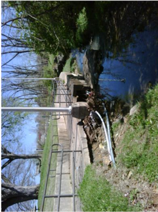
Figure 16a. Sidewalk area prior to 2009 repairs
